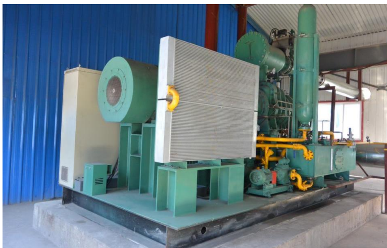
Fig. 2: steam expander KES600 installed at Tianfeng power plant No. 1
