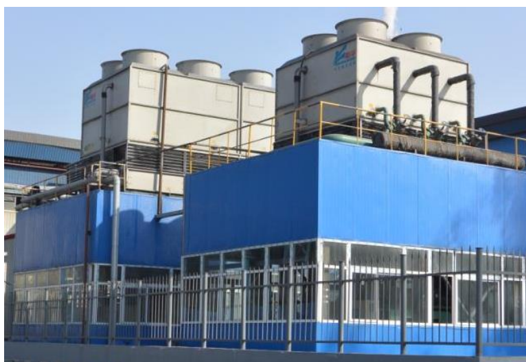
Fig. 3: ORC units installed at Tianfeng power plant No. 1
