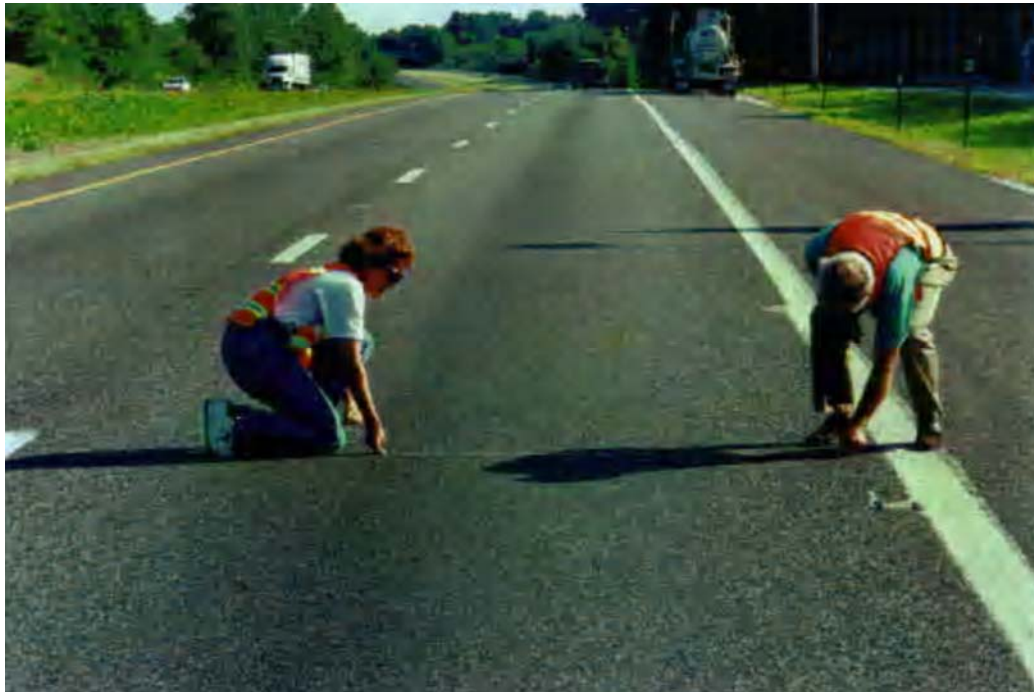
Figure 2: Rutting Measurement (after (8))
