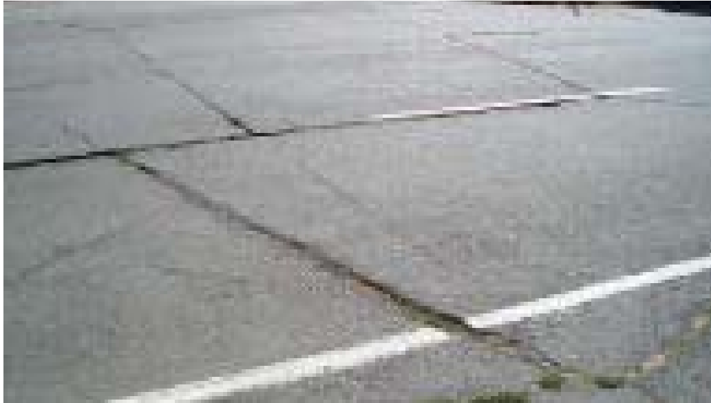
Figure 4: Reflective Cracking (after (8))
