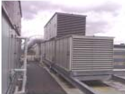
Business air conditioner
