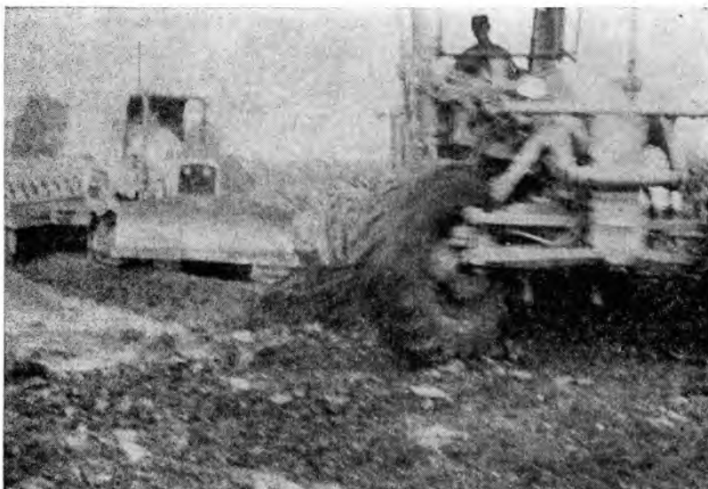
Figure 2. A motor grader and dozer-towed sheepfoot roller aid the chemical breakdown by providing both mixing and crushing action.
