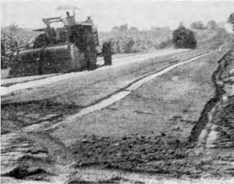
Figure 3. AC 20 applied to the recycled base by a distributor and thoroughly blended with a pulvimixer gives additional strength to this arterial road.
