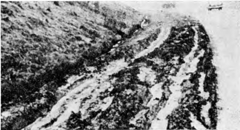
Figure 7. Problem indicator—wheel tracks in shoulder.
