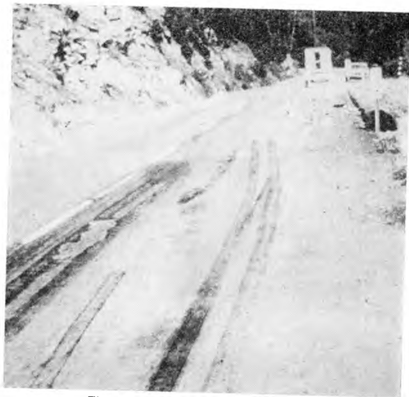
Figure 9. Problem indicator—skid marks.
