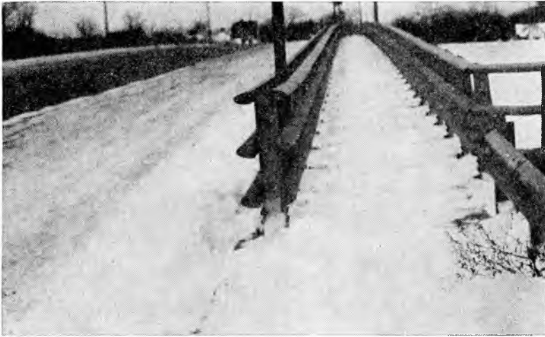
Figure 5. Attempt to protect heavy pedestrian movement—at potential hazard to vehicles—better end treatment possible.
