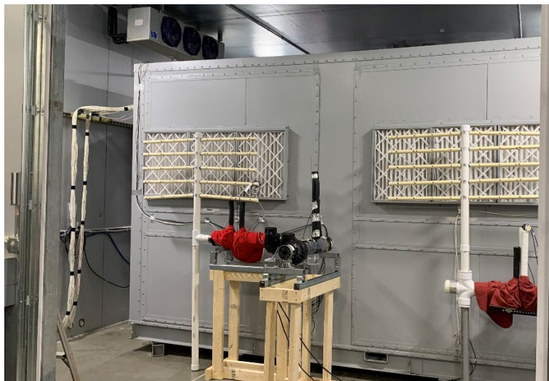
Figure 2: DOAS unit in psychrometric room. Psychrometers shown on regenerator (left) and conditioner (right) inlets.
