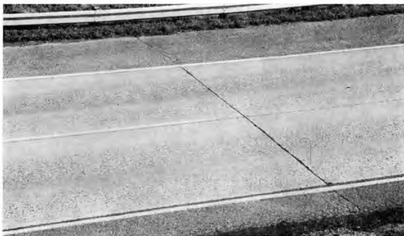
Figure 1. This is a Portland cement concrete pavement with gravel aggregate after five winters of studded tire traffic—approximately 10,450 ADT per lane—estimated 1.7 million total studded tire passes.
