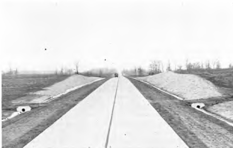
U. S. 31 By-Pass around Columbus. Note the wide shoulders and the flat cut-slopes, seeded and mulched for quick vegetation growth.
