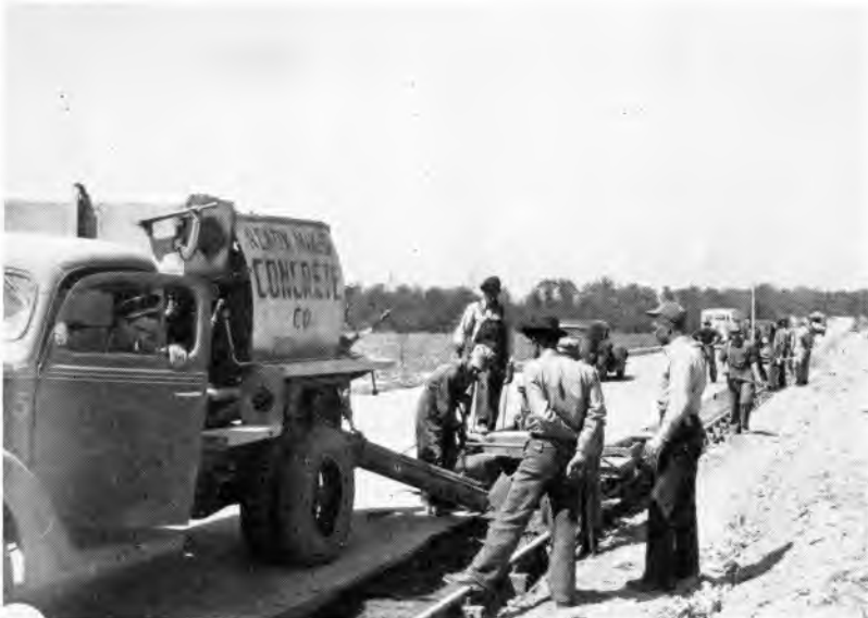
Roads carrying considerable truck and bus traffic should have traffic lanes of eleven feet. This is a section of U.S. 31 south of Scottsburg receiving a concrete widening strip.
