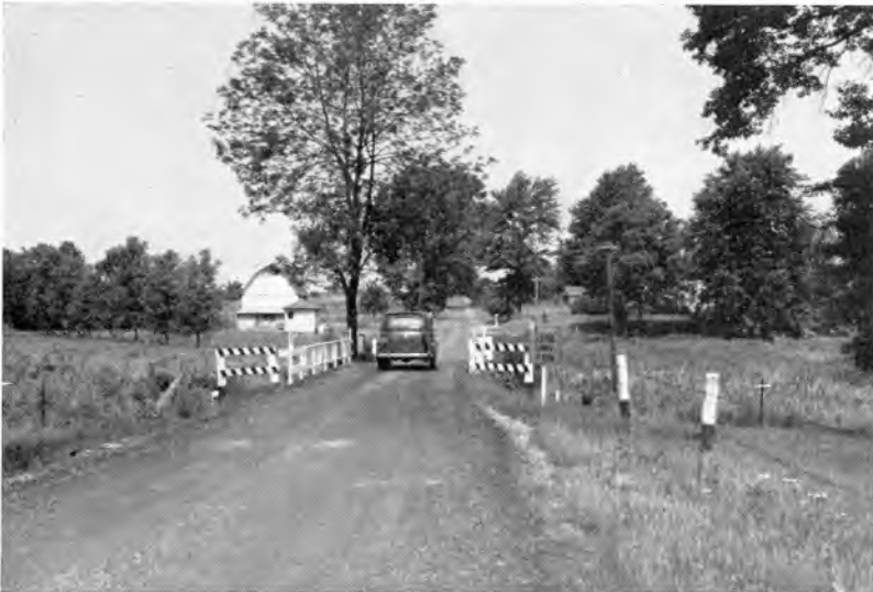
Hundreds of narrow bridges and culverts, many with very limited load-carrying capacity, are handicapping the free and safe movement of traffic.
