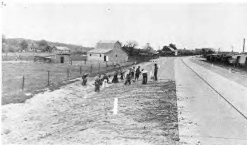
Shoulder widening and finishing along State Road 67 near Gosport. Note flatter slope from wide shoulder into and beyond ditch line made possible by wide right-of-way.
