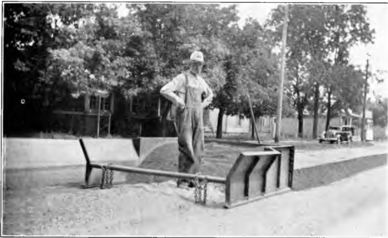
Fig. 1. Combining old and new aggregate into a uniform windrow by use of the "Proportioner".
