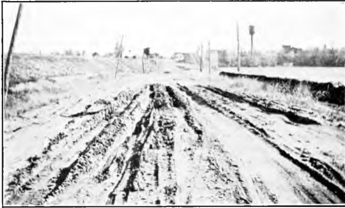
Fig. 8. Road softened by seepage.
