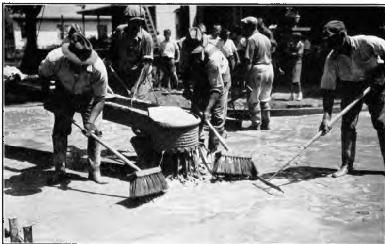
Fig. 2. Grouting and brooming. Note attachment with perforated bottom on end of chute to break up impact of grout on surface.
