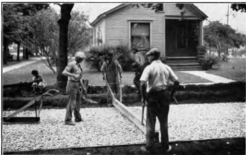
Fig. 1. Final tamping before grouting, and correction of irregularities in surface by use of template.
