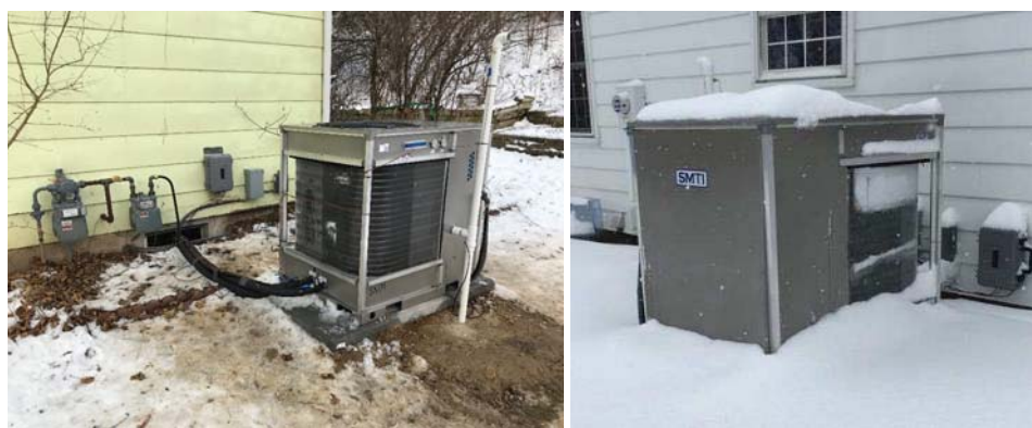
Figure 1: Pre-commercial GAHPs operating at WI demonstration sites
