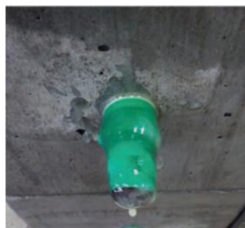
Figure 3. Insulated end of steel bar during corrosion.
