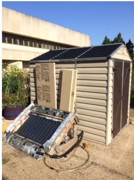
Figure 3 Solar collector with glazing connected to a heat exchanger contained in the outdoor facility
