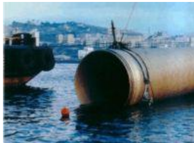
FIGURE 1 EXAMPLE COMPOSITE PIPING OFFSHORE
