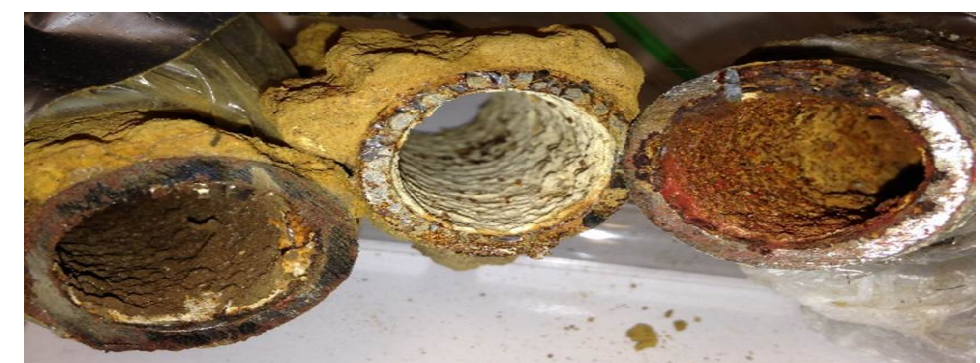
Figure 2. Different kinds of iron corrosion and rust found in Flint drinking water pipes. Photo credit: Min Tang and Kelsey Pieper. (Panko, 2017). Smithsonianmag.com
