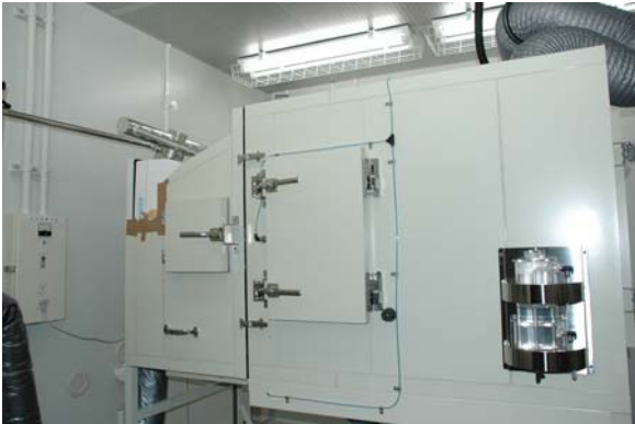
Figure 2: Indoor-unit room (air chamber)
